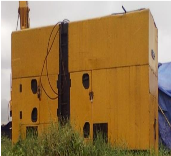
Genset MITSUBISHI/S6A-PTA/380 KVA, in POOL/G.PUTRI/BOGOR.
