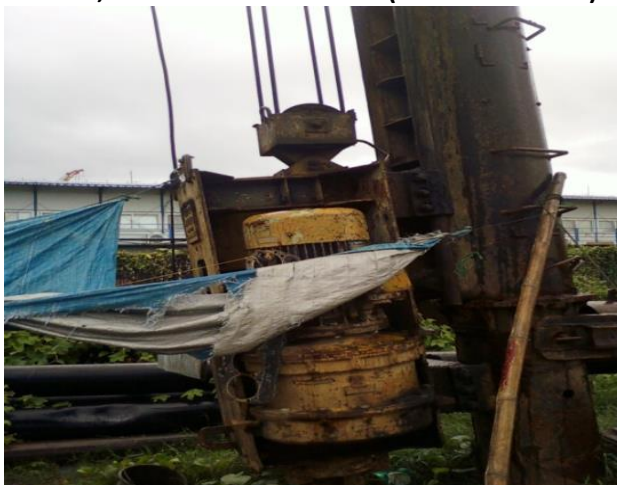
SANWA Motor 45KW/45KVA, in POOL/G.PUTRI/BOGOR.
