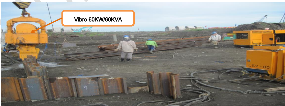
Vibro TOMEN/60KW/60KVA, in ADIPALA/CILACAP.
