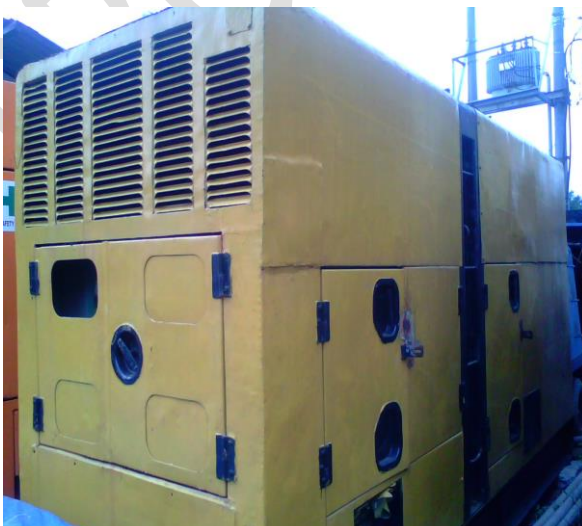
GENSET MITSUBISHI 380 KVA, In POOL/G.PUTRI/BOGOR
